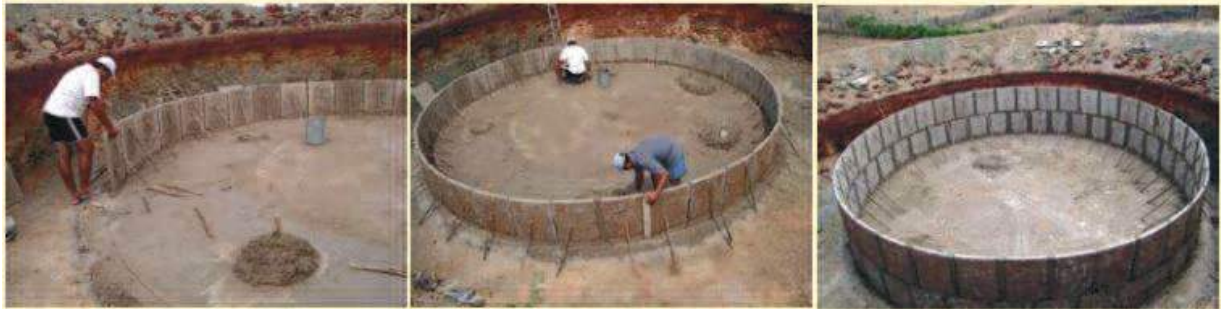
Figure 5 Constructing a 52m 3 tank with concave cement plates (ASA 2011), catchment area for such a tank is shown at right
